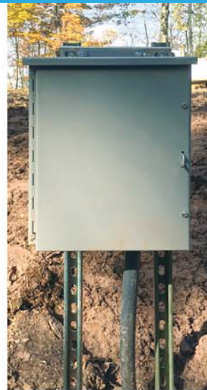
Multiple cable-drops of installed sensors can be manually accessed above grade with a tablet PC and dataPIMS™.
